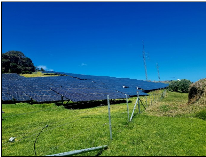
Solar farm, a major part of the island power supply.
